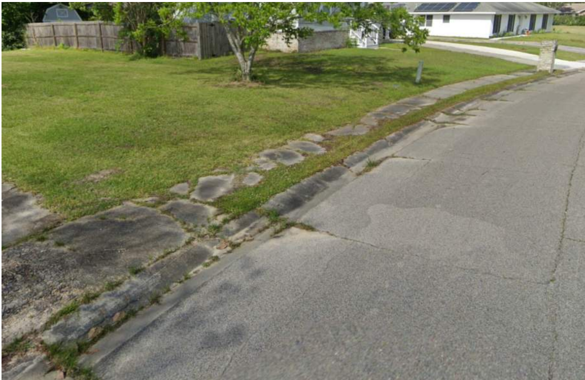
Figure 5: Damaged Pedestrian Access Route
