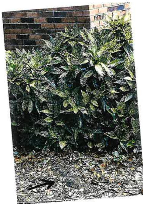
LARGE ROOT EXTENDING UNDER SOUTHWEST CORNER OF FOUNDATION
