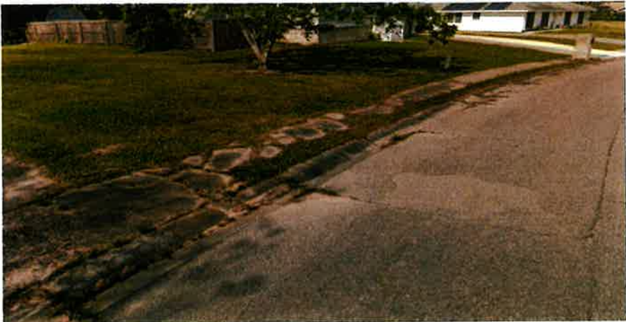
Figure 5: Damaged Pedestrian Access Route
