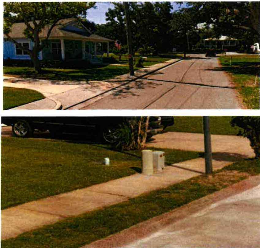
Figure 1: Obstruction Within Pedestrian Access Route
