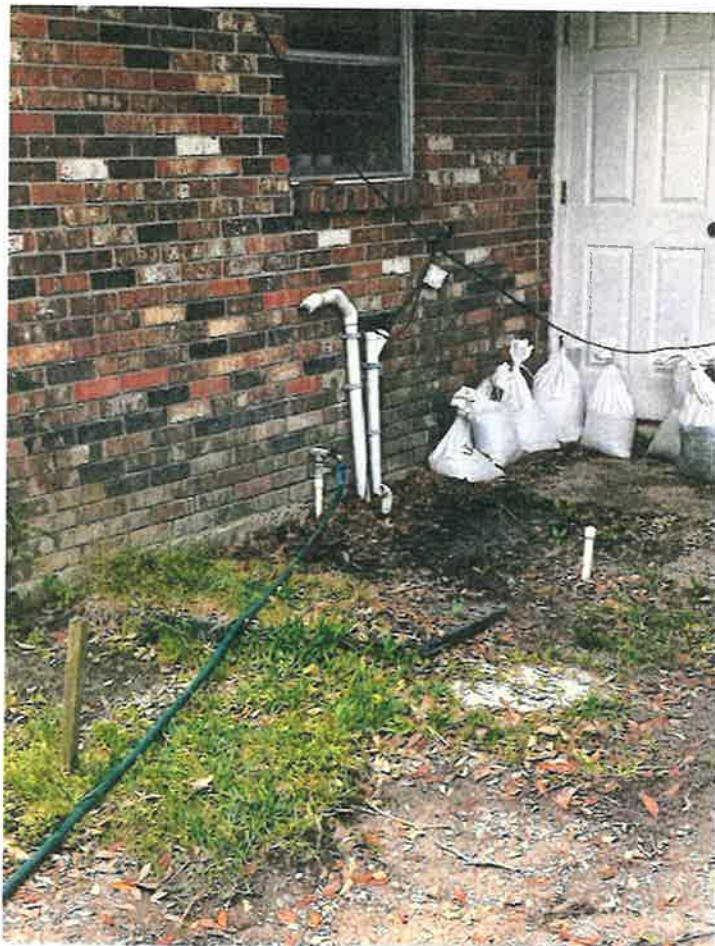
Pic of Kitchen Plumbing due to Tree roots
