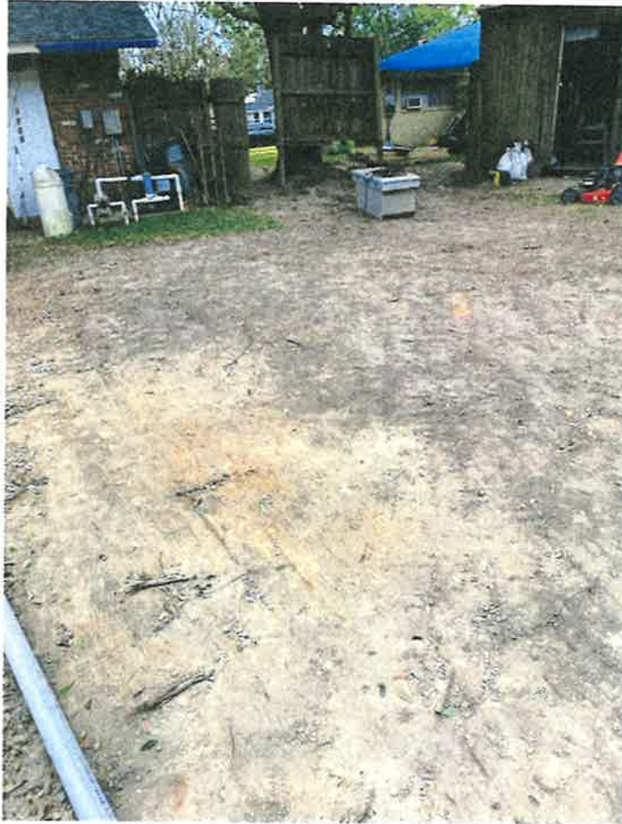
Tree roots throughout the yard
