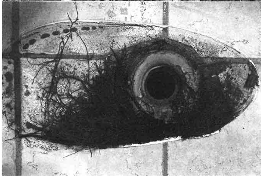
plumbing issues caused by Tree 1
