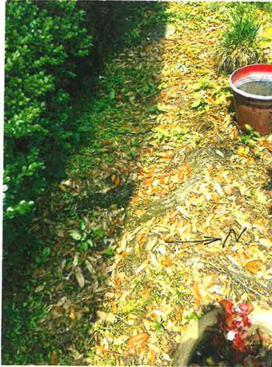
BIG ROOT GROWING UNDER HOUSE FOUNDATION
